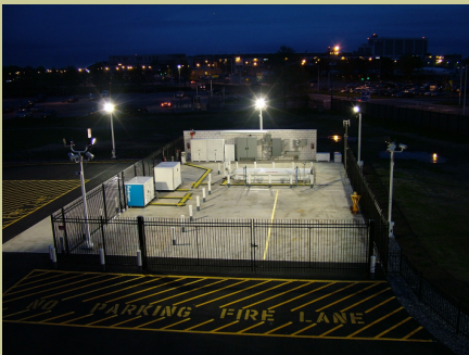
UHF JFK Hydrogen Filling Station
